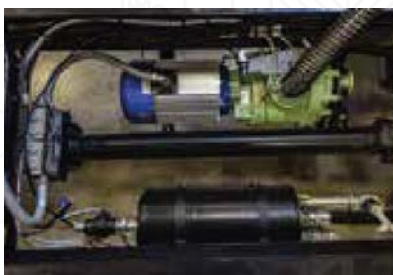
PTO DRIVEN COMPRESSORS AND GENERATORS
